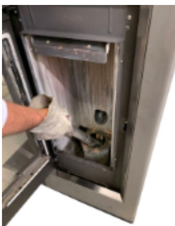
Fig. 33 - Burning pot box cleaning
